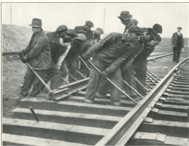
A picturesque operation is the placing in exact position of a new rail on the leveled cross ties
